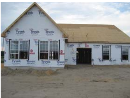
Progress is going very well for Sgt. Jason Neilson's home in Milford, DE thanks to LaCrosse Homes
