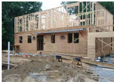
Progress on the home being built in Wharton, NJ for Spc. James Benoit
